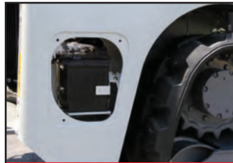
Battery Access Panel
